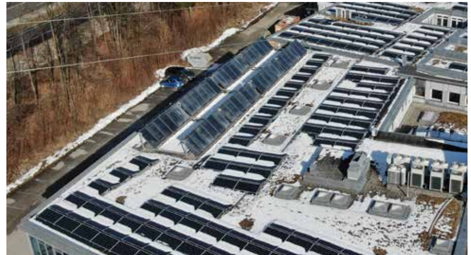
Installation of solar power reduced energy usage at Besi Austria
